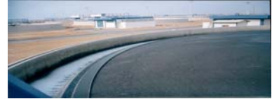
Primary Sedimentation Tank
