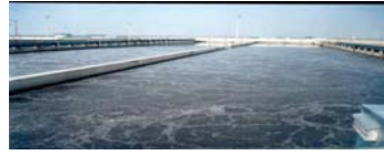
Oxidation Ditch Tank
