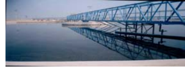
Final Sedimentation Tank
