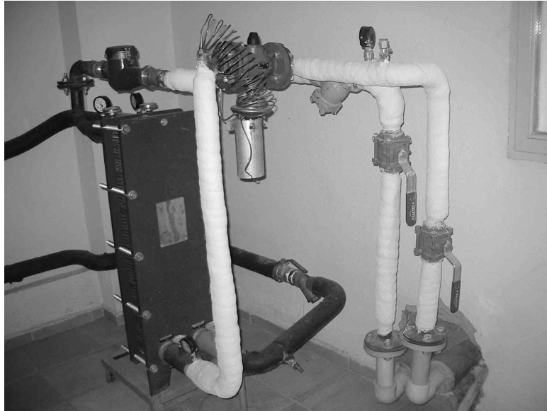
Figure 6.3. Heat exchanger and the flow meter at the Ardiç apartment building
