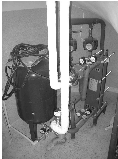
Figure 6.4. Heat exchanger and the flow meter at the Doğan apartment building
