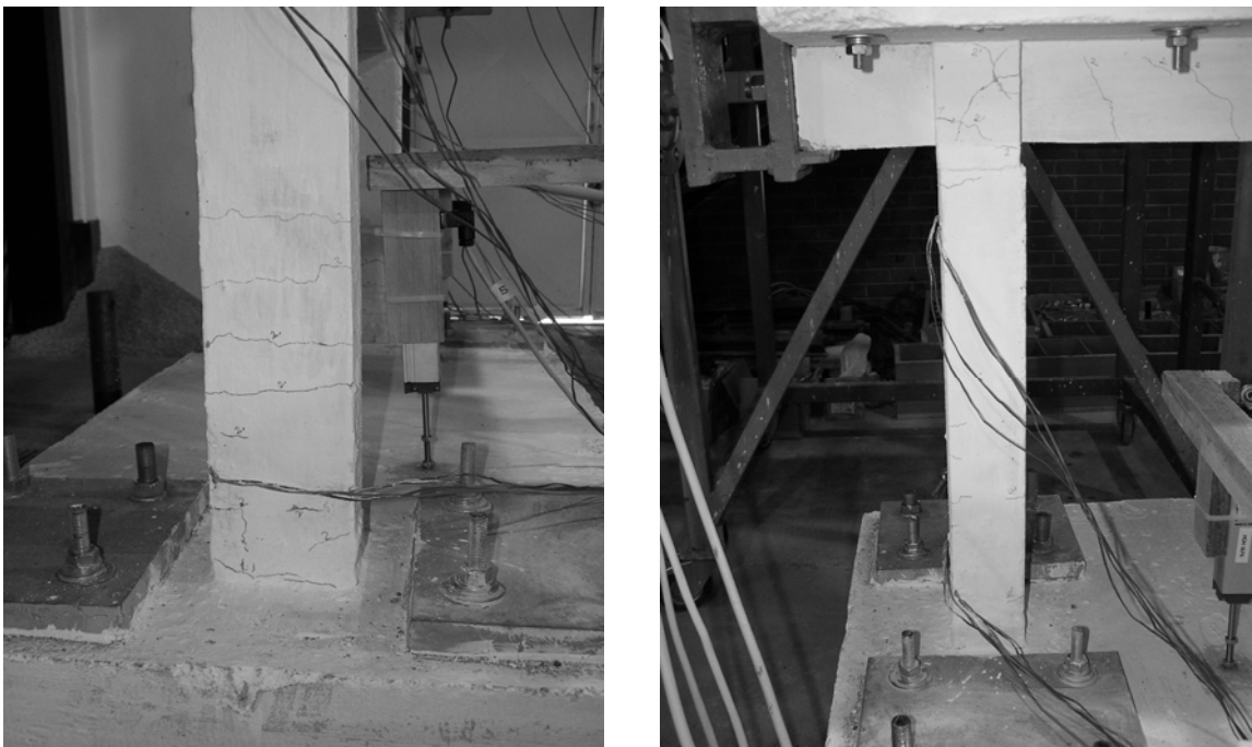
Figure 3.10. Flexural cracks at the east face (left) and shear cracks at the north face (right) of the first story east column at the end of the second loading group
