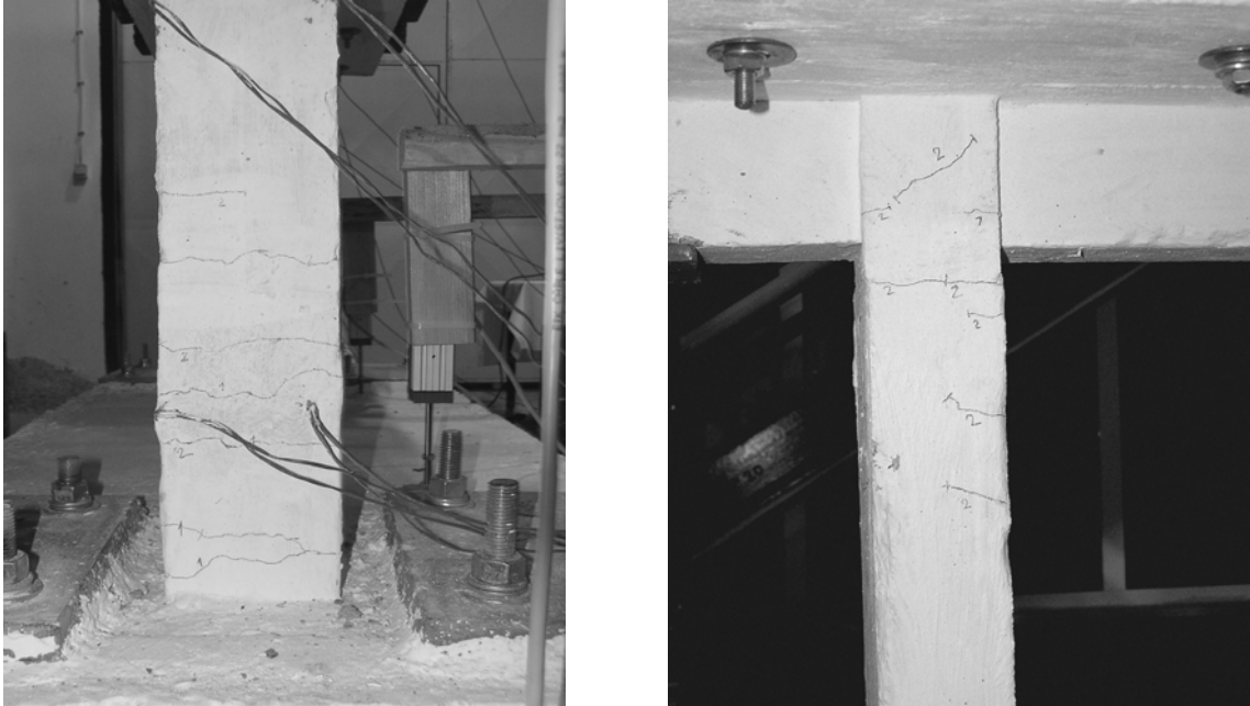
Figure 3.14. Spreading of flexural cracks at the east face of the first story east column (left) and new shear crack in the joint zone of second story north face east column (right) at the end of the second loading group
