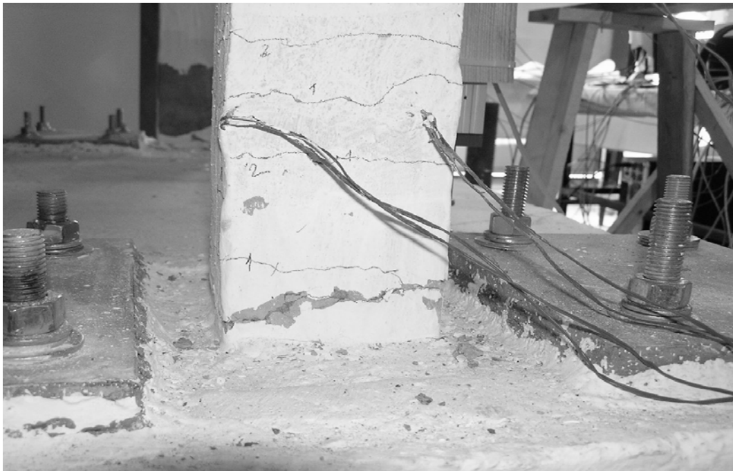
Figure 3.16. Crushing of concrete on the first story, east face of east column, end of the fourth loading group
