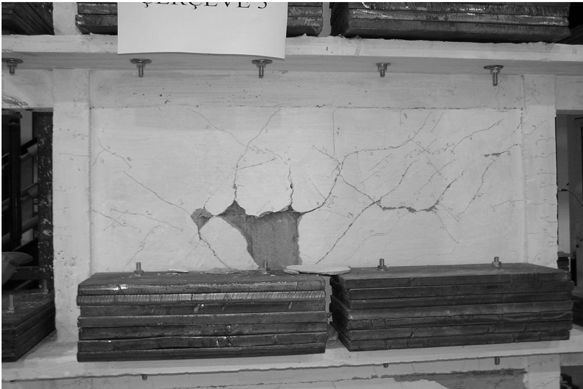
Figure 3.22. Spalling of the partition wall plaster in the second story north face
