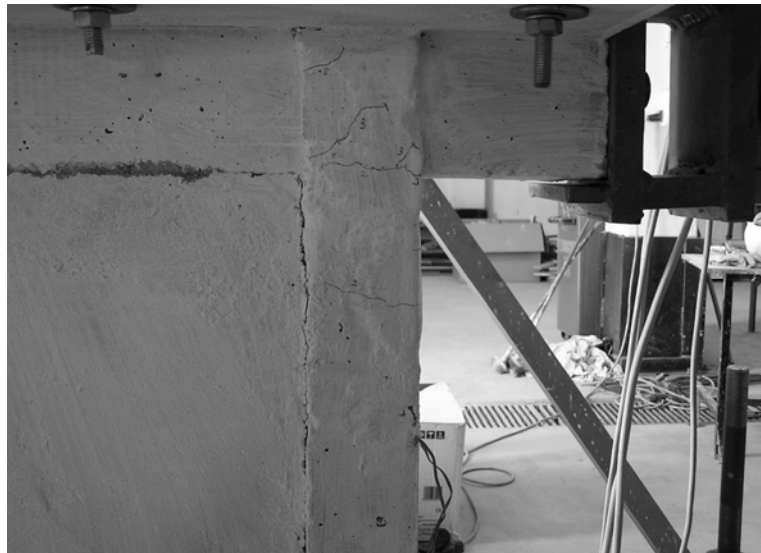
Figure 3.28. Damage in the joint zone of the first story at the end of third loading group, east column
