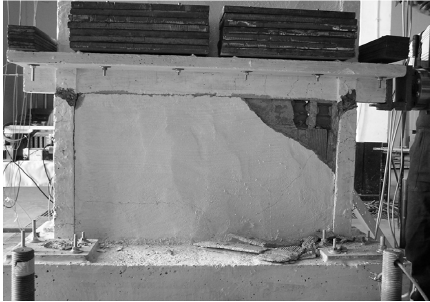
Figure 3.30. Damage of the first story at the end of the sixth loading group, south face
