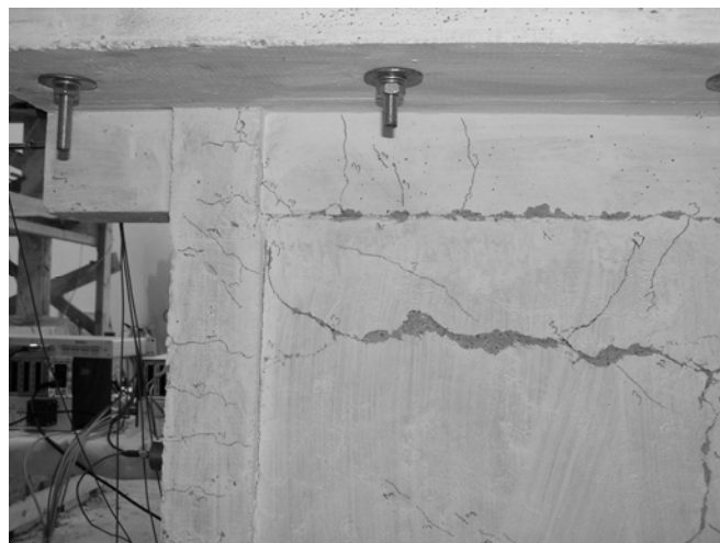
Figure 3.21. Flexural and shear cracks in the first story beam at the south face, at the end of the third loading group
