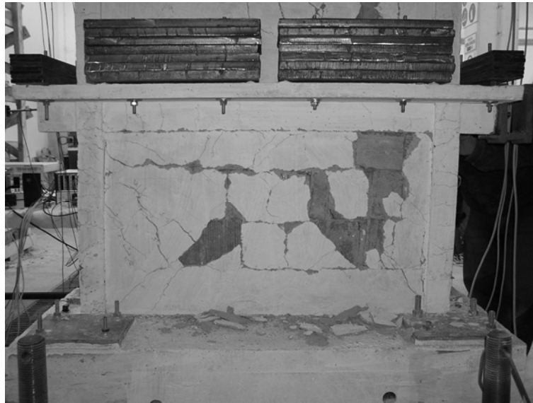
Figure 3.23. Residual deformation of the first story columns and the partition wall
