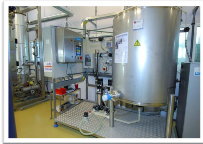
Figure 4.7. De-ionised water treatment unit
