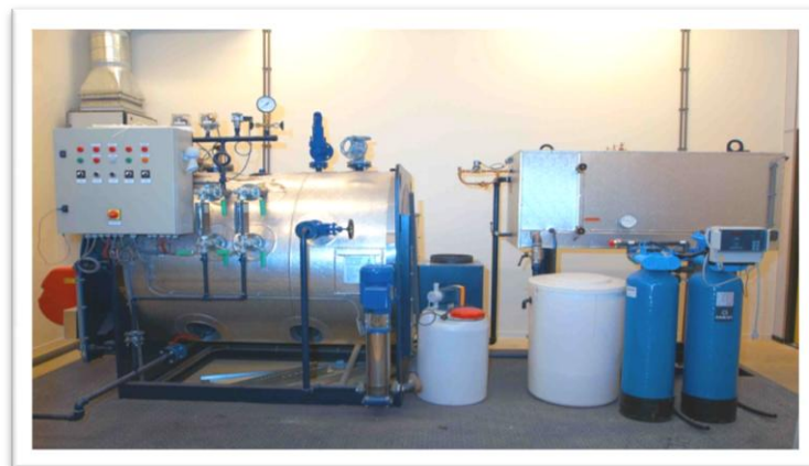
Figure 4.8. Gas boiler unit
