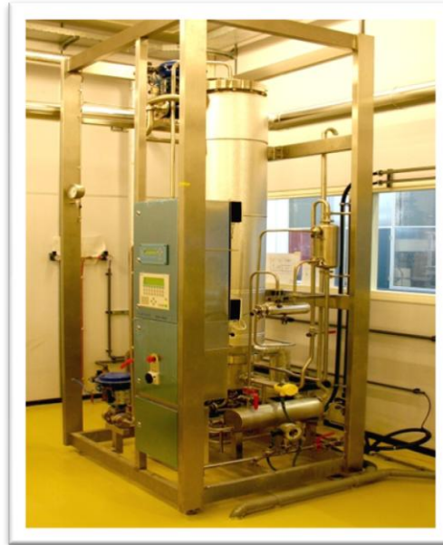
Figure 4.9. Clean steam generator unit
