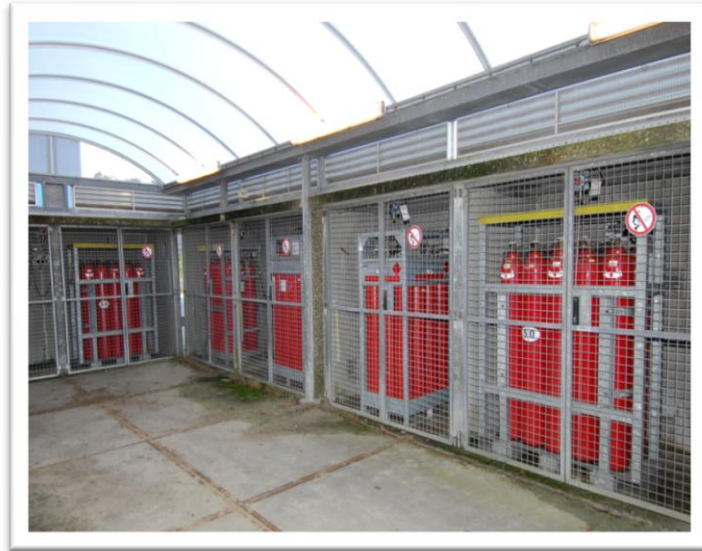
Figure 4.5. Gas bottle storage and distribution room
