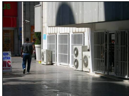
Figure 4.13. A view from an air cond. installment at street level
