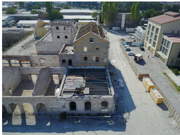
Figure 88. Roof system of Building 3 undergoes enforcement during the restoration process (Source: Grid İnşaat)
