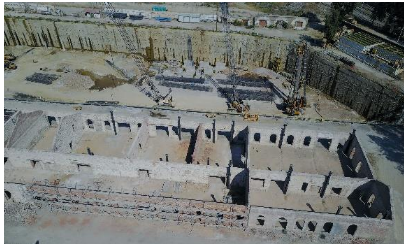
Figure 80. During the restoration works, enforcement studies are carried out on the wall systems of Building 1 and 2 (Source: Grid İnşaat)
