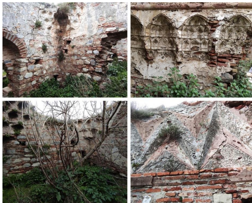
Figure 3. 11. Structure failures and material deterioration of Kale Altı Bath: Structure failures and material deterioration (probably due to weather conditions, rainwater penetration, rising damp, lack of maintenance, seismic forces, or vandalism): Joint discharge (a), Discoloration (b), Plant growth (c), Microbiological colonization (d)
