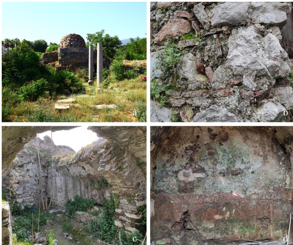
Figure 3. 8. Structure failures and material deterioration (probably due to weather conditions, rainwater penetration, rising damp, lack of maintenance, seismic forces, or vandalism): Plant growth (a), Joint discharge (b), Discoloration, (c), Microbiological colonization (d)
