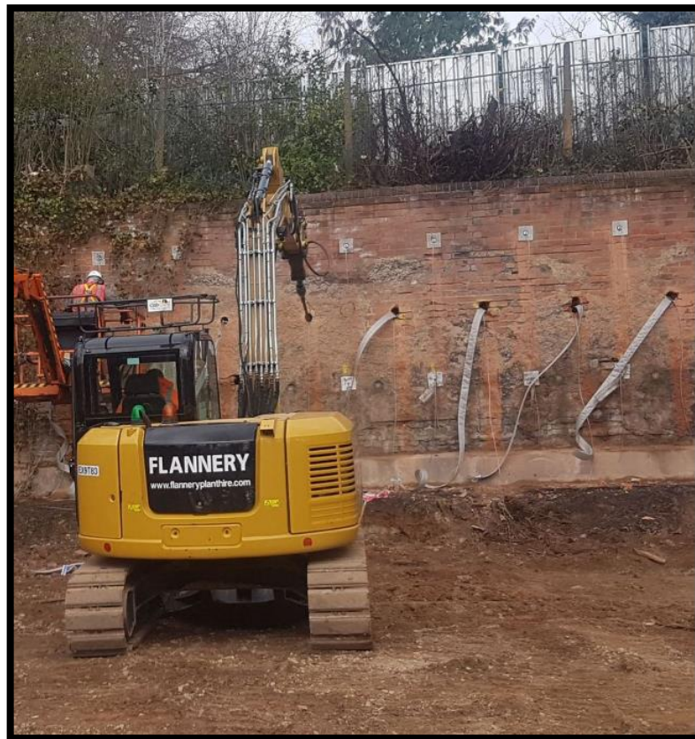
Figure 2.35 Reinforcement of existing retaining wall with flip anchors England (Source: Platipus Civil Engineering & Construction Brochure, 2022)
