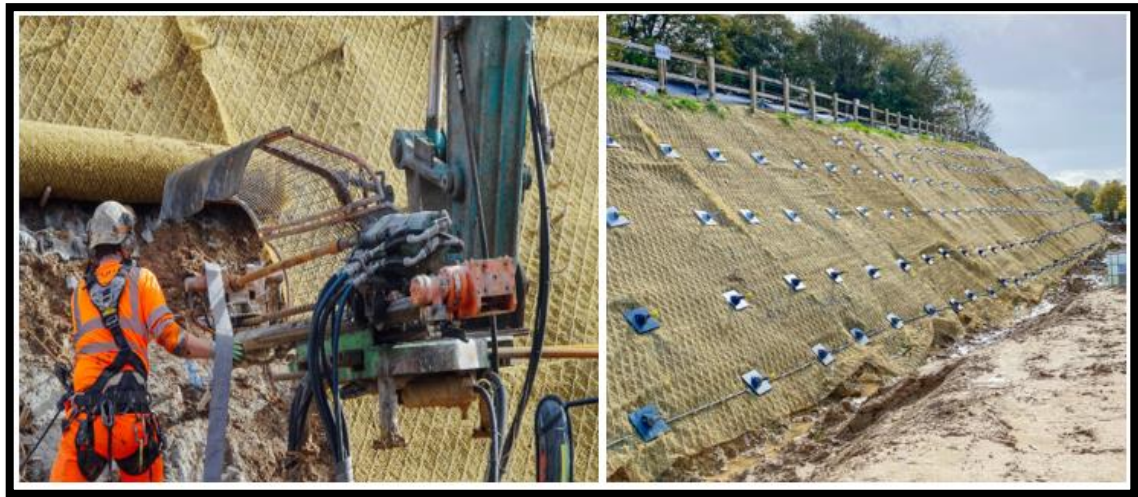
Figure 2.32 Flip anchor applied to a soil-covered hillside in Stubbington England (Source: Anchor System International, 2020)
