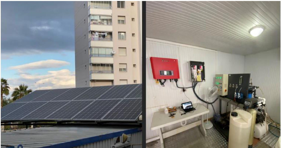
Figure 13. Reverse osmosis and PV systems of the geothermal heat center in Yenikale (Tomaszewska et al. 2021)
