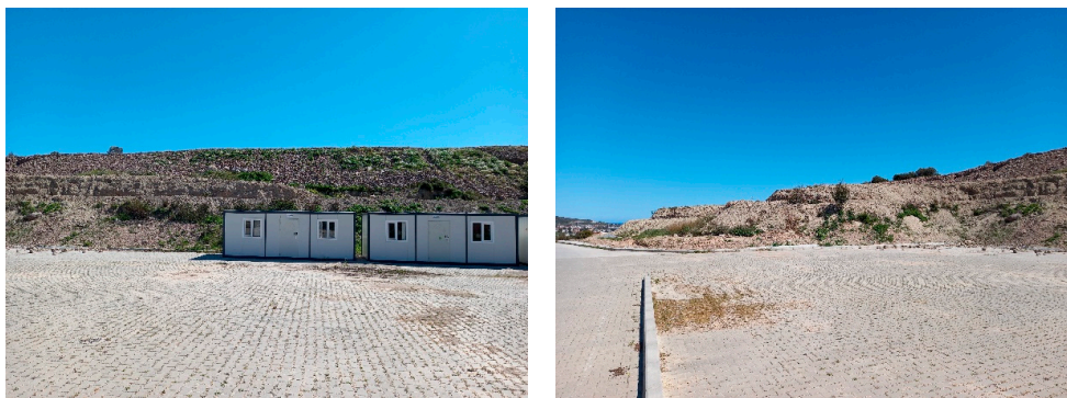
Figure 9. Erosion along the Rectorate Road.
