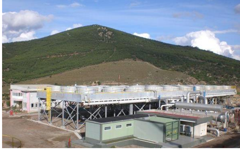
Figure 2. 4. Tuzla Geothermal Power Plant located in Çanakkale, Ayvacık (Türkiye)
