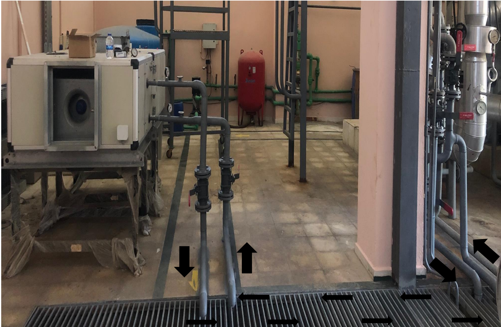
Figure 4.8. Dryer-geothermal line connection
