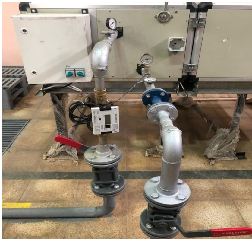
Figure 4.7. The inlet-outlet line of the geothermal fluid to the dryer
