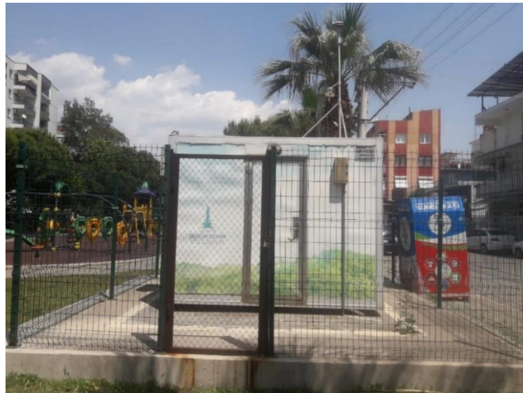
Figure 5.3. Picture of Bayraklı air quality monitoring station. (Source: taken by the author)
