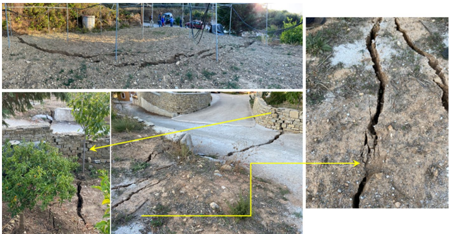
Fig. 24 Ground and pavement cracks in the village of Kontakeika (Samos), indicative of the mobilization of an extended but mild slope or more broadly characterized as seismically-induced secondary ground failures. The cracks extended on both sides of the street through soft soil formations. Arrows in the figure explain the relative location of the cracks
