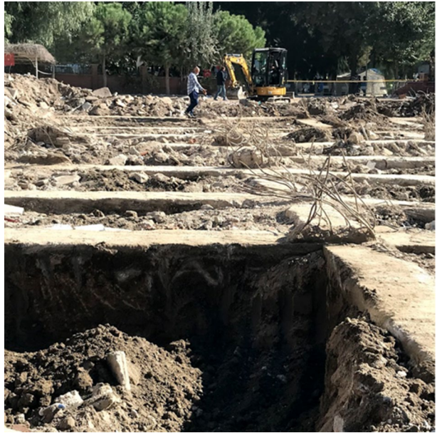
Fig. 2 Two-way combined footing system (grid spread footing foundation) of one of the heavily damaged buildings in Bayrakli, whose collapse is not foundation induced
