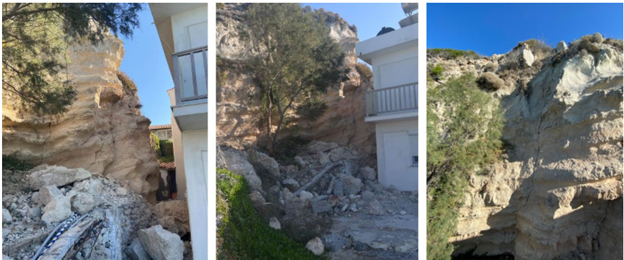
Fig. 22 Detachment of sandy marls and marly limestones recorded very close to a residential building in the Kokkari region (photos taken by the HAEE/ETAM reconnaissance team, 37°46'49.9" N, 26°53'35.0" E). Vertical open cracks are visible, clearly susceptible to detachment and toppling
