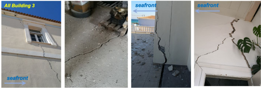
Fig. 17 Building affected by lateral spreading towards the seafront in the neighborhood of Vyrsopepsia in Karlovasi ( 37^{\circ}48'01.1'' N 26^{\circ}42'20.6'' E). The cracks observed running across the building indicate 3–5 cm of movement [photos courtesy of Prof. K. Antonopoulos]
