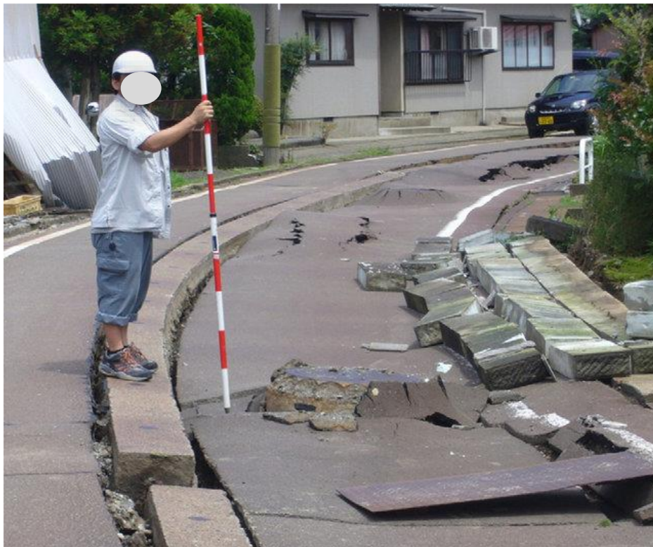
Figure 2.11. Uplifted manholes and settled backfill after the Noto Peninsula Earthquake, Japan, 2007 (Mw=6.9) (Kang et al., 2013)
