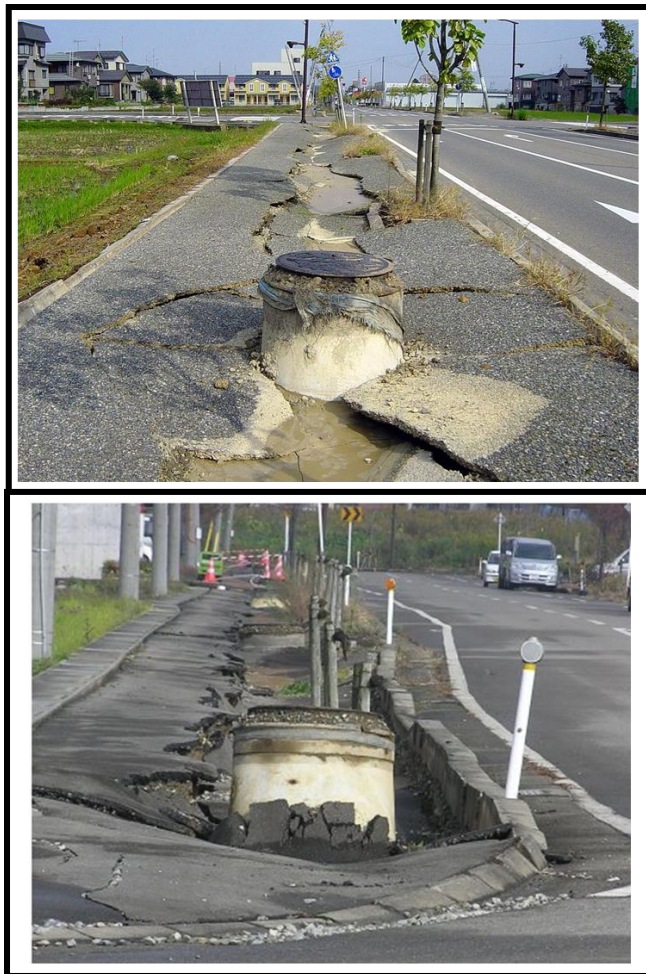
Figure 2.9. Uplifted manholes and settlement of sidewalks after the Earthquake in Niigata-ken Chuetsu, 2004 ( M_w=6.6 ) (Kang et al., 2014b)
