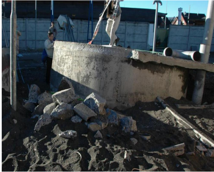
Figure 2.8. Uplifted sewage tank after the Maule-Chile Earthquake, 2010 ( M_w=8.8 ) (Kang et al., 2014a)
