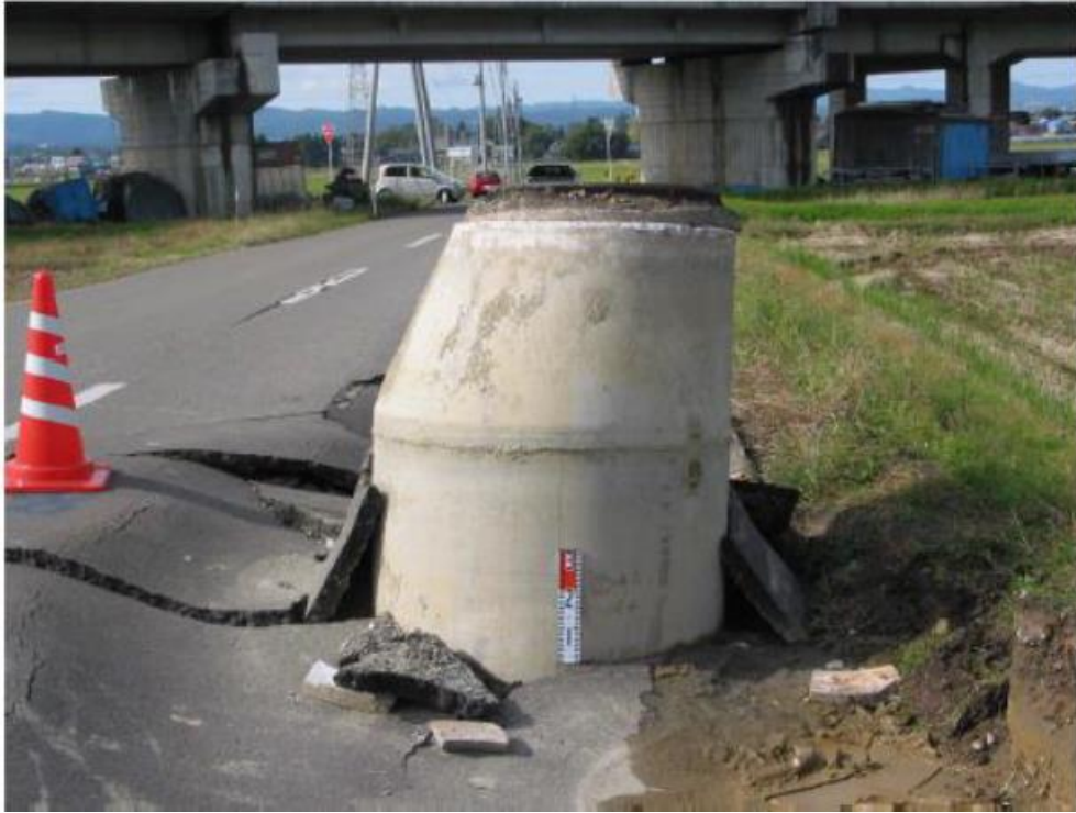
Figure 2.10. Uplifted manhole after the Earthquake in Niigata-ken Chuetsu, 2004 (Mw=6.6) (Tobita et al., 2009)
