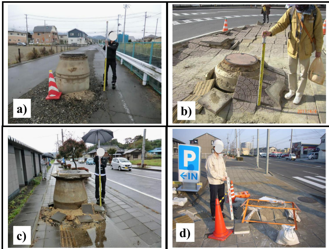
Figure 2.7. Uplifting manholes during Pacific Coast of Tohoku Earthquake, 2011 ( M_w 9.1) a-c) sewage network manholes, d) rainfall network manhole
