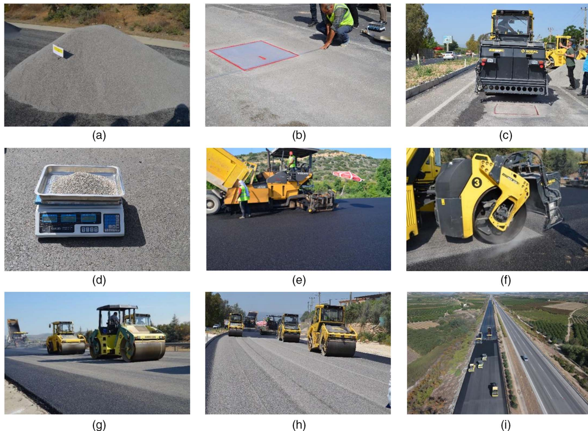
Fig. 2. Photographs taken during gritting application on working sites: (a) stockpiled gritting aggregate; (b) preparing the laying area; (c) adjusting spreader; (d) determining the spreading rate of aggregate; (e) construction of the SMA; (f) gritting application; (g) compaction of the gritted sections-1; (h) compaction of the gritted sections-2; and (i) general view of construction site. (Images by İslam Gökalp.)
