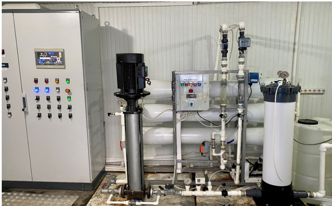
Figure 9. Large pilot-scale NF/RO treatment system.
