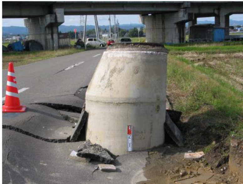
Figure 1.2. Uplifted manhole after the 2004 Niigata-ken Chuetsu, Japan, Earthquake (Source: Tobita et al., 2009)
