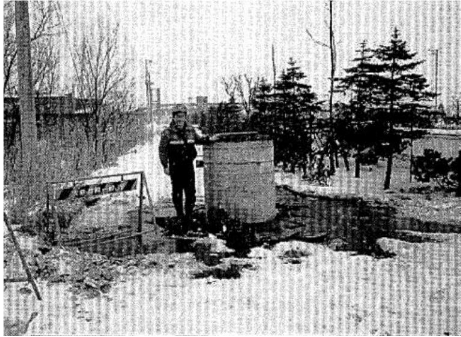
Figure 1.1. Uplift of manhole after the 1993 Kushiro-oki earthquake in Kushiro Town (Source: Yasuda and Kiku, 2006)
