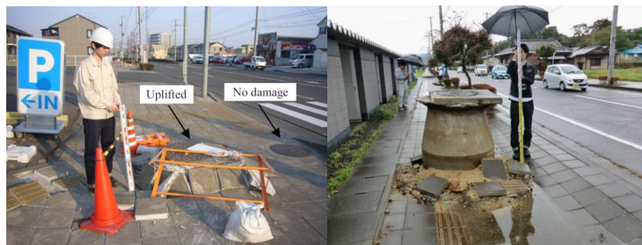
Figure 1.4 Right: Uplift of a manhole at Shiraishi, Left: Uplift of a manhole at Iwakiri (Source: Yamaguchi et al., 2012)
