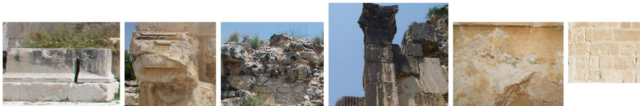
Figure 21. Mapping of the weathering forms of stones used in the triumphal arch (Alakapı)
