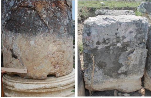
Figure 16. Exfoliation and spalling observed on stone surfaces.
