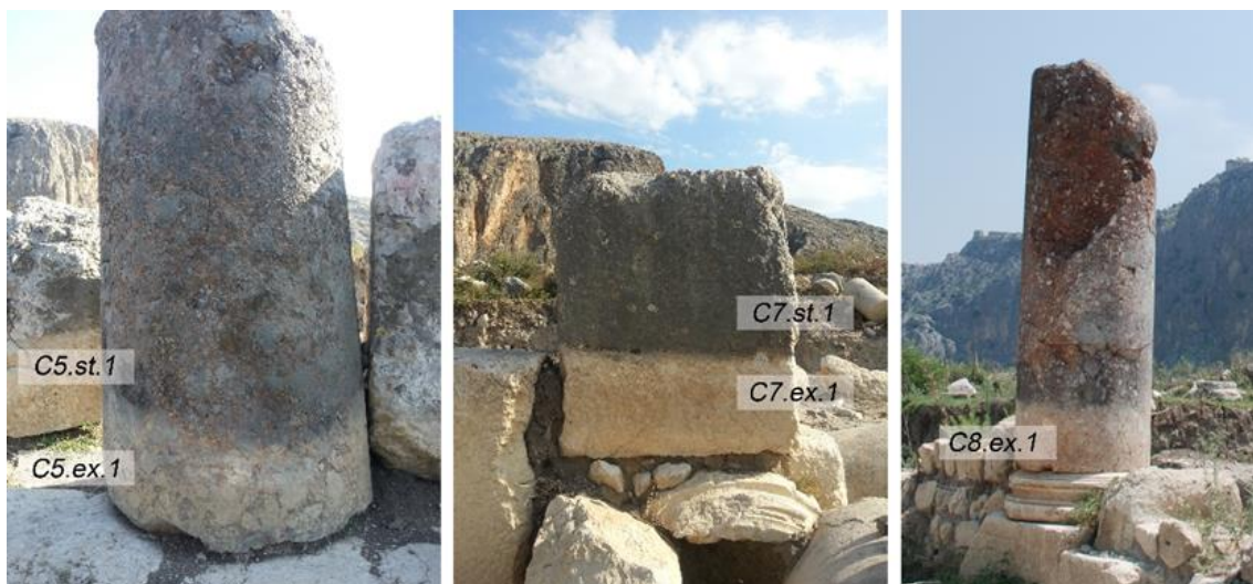
Figure 69. Samples from standing and recently excavated surfaces of the 5 th , 7 th , 8 th columns.
