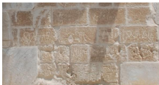
Figure 19. Stretch observed on stone surfaces.
