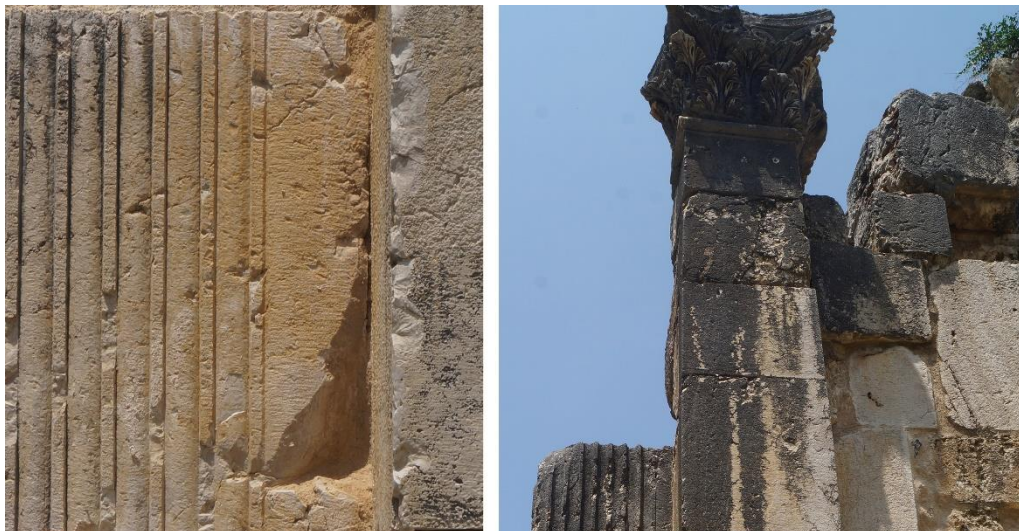
Figure 15. Yellow patina and black crust observed on the stone surfaces.
