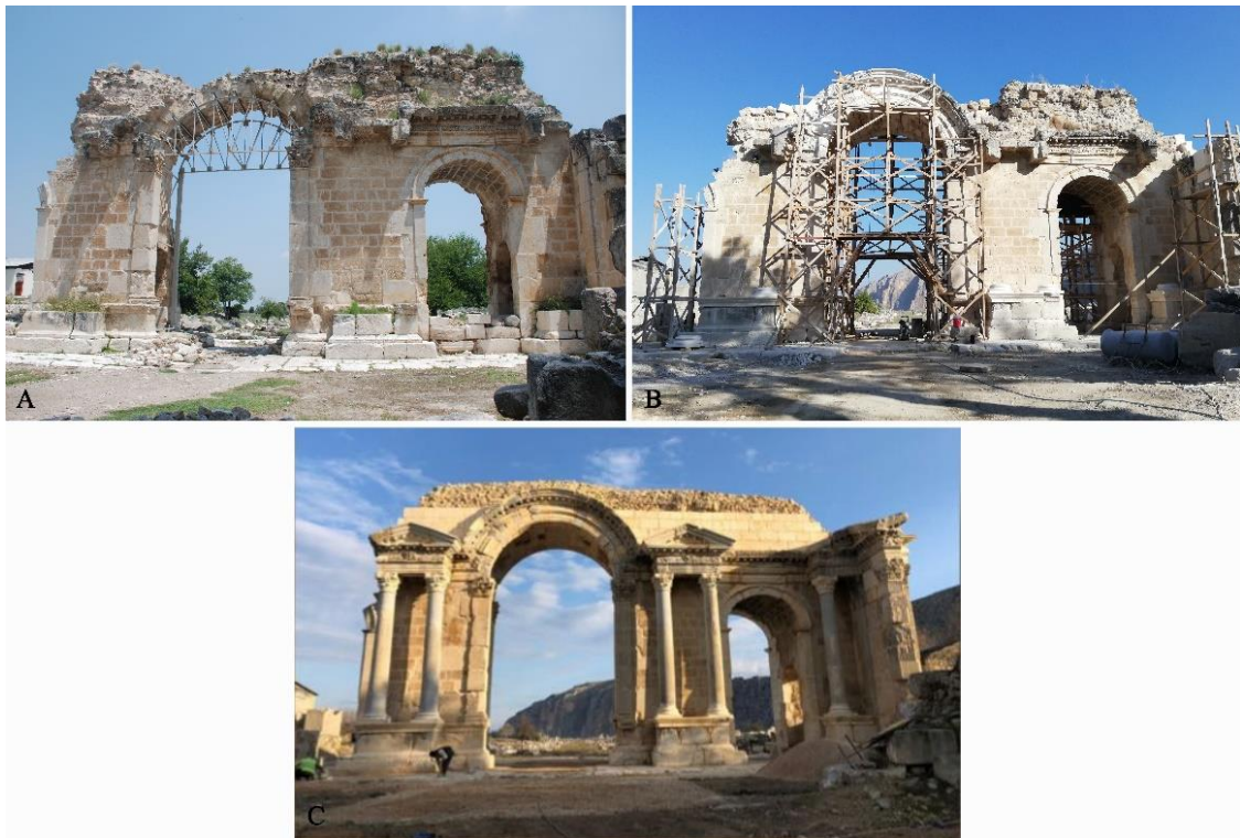
Figure 10. The images of the triumphal arch (Alakapı); in 2018 (A), during the restoration works in 2019 (B) and after restoration in 2020 (C).
