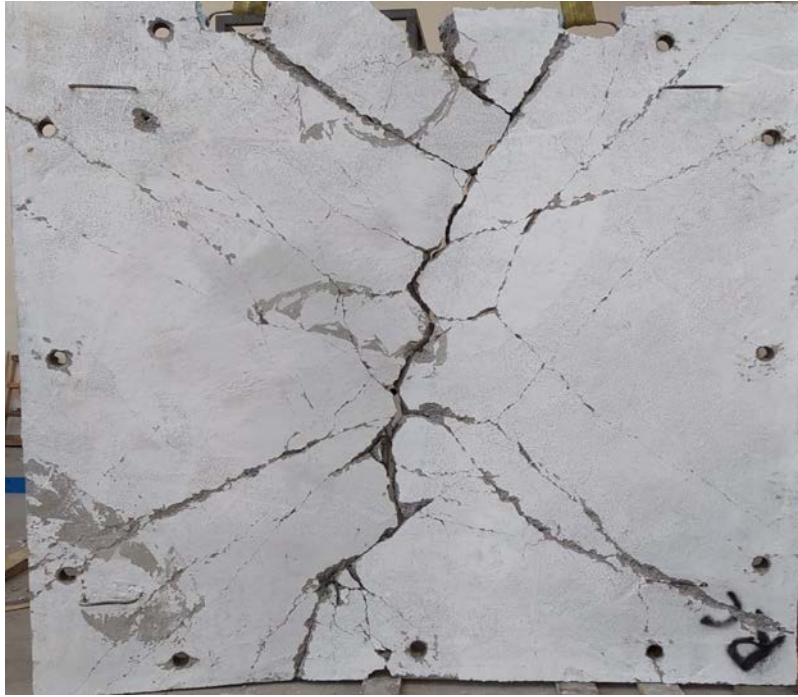
Figure 4.4.23. Front Face Crack Patterns After Testing for Panel JA-Plain-RF
