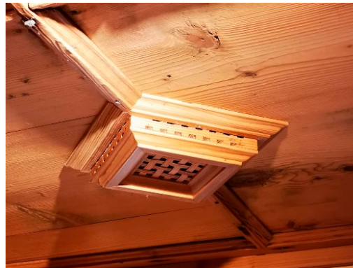
Figure 9. Integration of an exhaust air opening in a typical suspended wooden ceiling as commonly found in Tyrolian farms. Source: Michael Flach. Spatial impact: Starting with the vertical hidden piping in the existing chimney, a solution for the air supply openings must be considered. Flat ducts can be integrated between the beams of the wooden ceiling and hidden by a second wooden cover at the bottom to match the look of the existing wooden soffit. An air intake opening coming directly from the unused chimney of the smoking chamber would also be a possibility if it is concealed by a suitable wooden grille.
