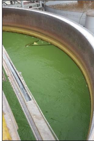
Figure 2. 11. MHP precipitation tank in Gördes HPAL Plant
