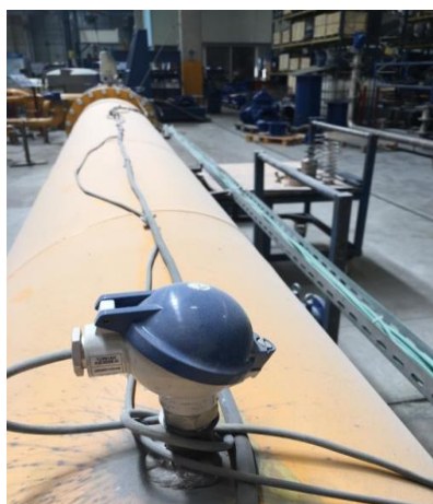
Figure 3.4 Water Temperature Measurement by a Thermocouple
