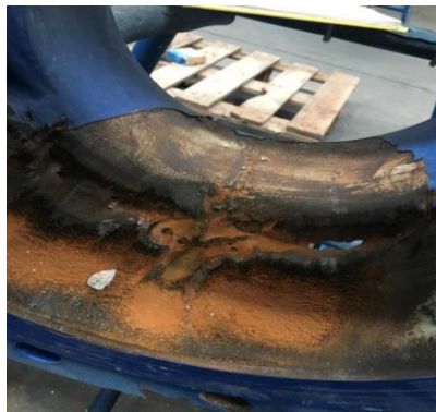
Figure 1.3: Effect of Cavitation on Valve Surface
