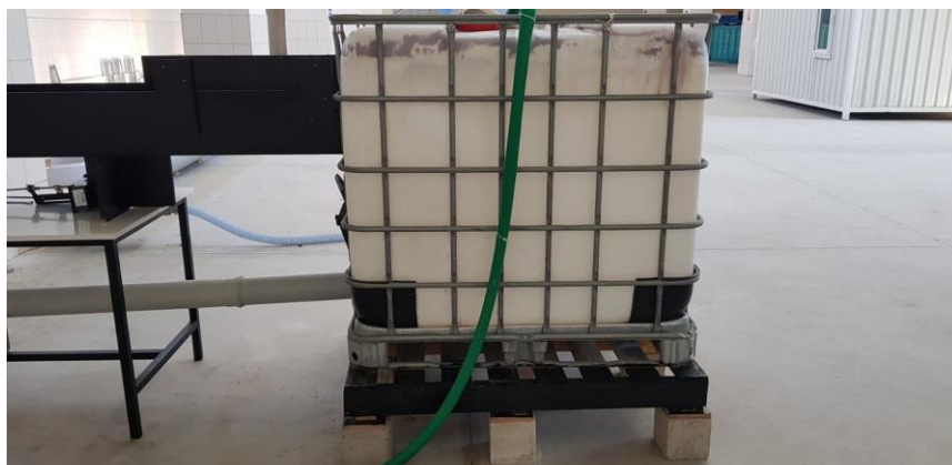
Figure 51. Image of energy dissipation tank
