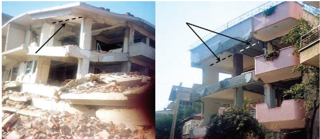
Figure 1.2. Damages related to frame discontinuity (Source: Bal & Ozdemir, 2006)
