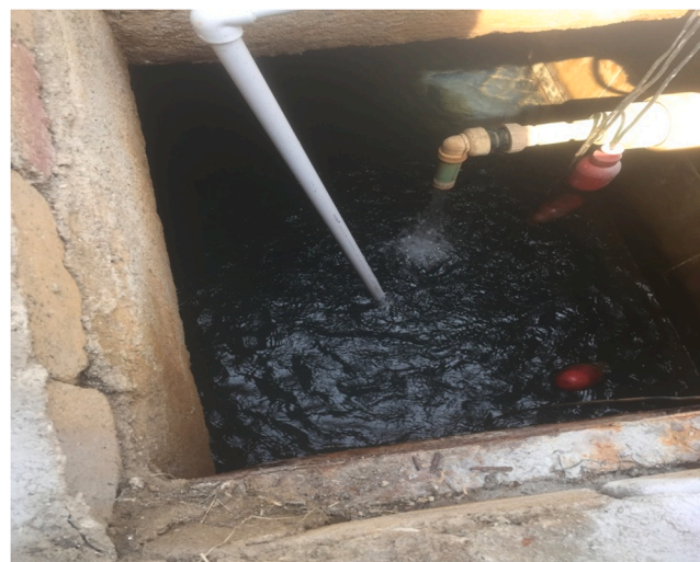
Fig. 2. Spent geothermal water reservoir.
